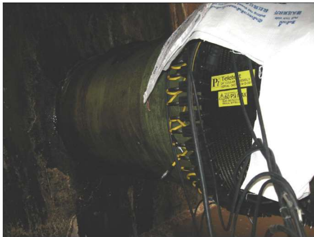
Multi Mode collar installed on pipe in chamber B. White plastic cover to prevent water ingress from leaks in concrete wall
