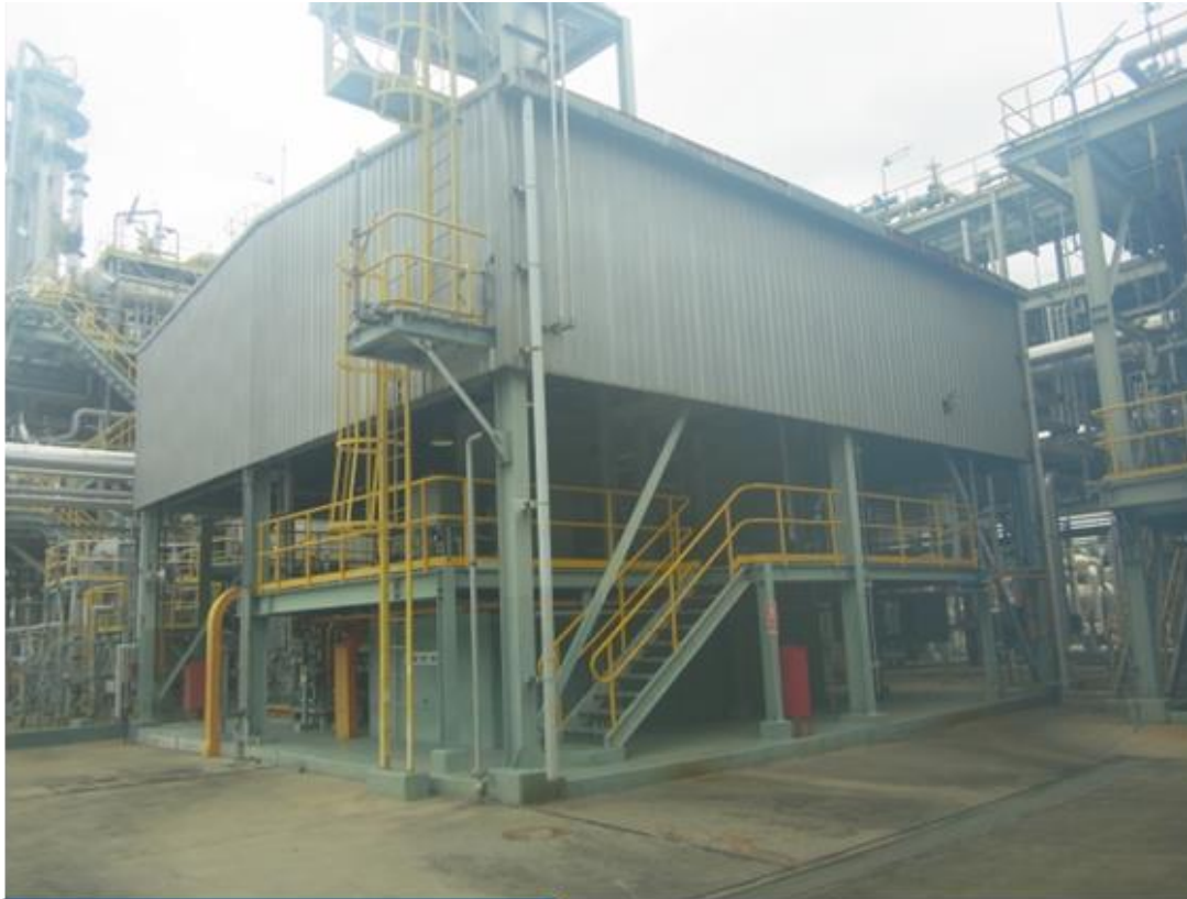
GSP.5 Regen Gas Shelter
