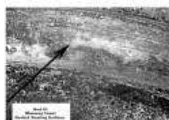
Figure B.53—Corrosion on Shell Weld Surface
