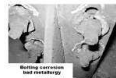
Figure B.16—Hardware Corrosion
