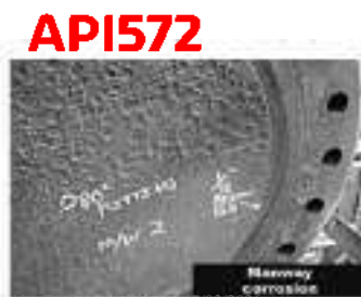
Figure B.51—Marine Corrosion
