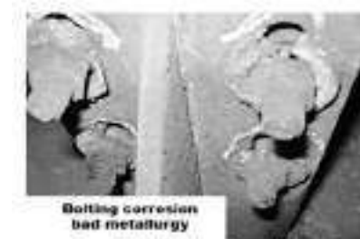
Figure B.48—Hardware Corrosion
