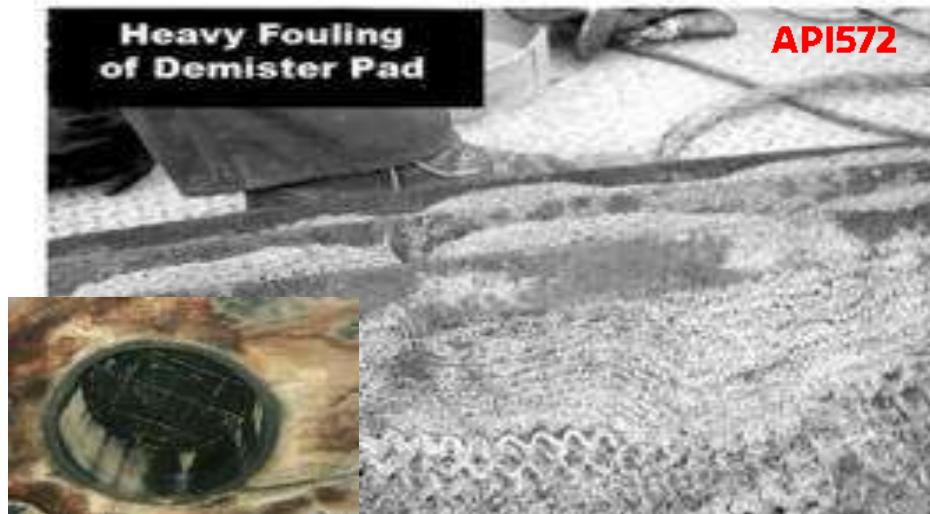
Figure B.39—Fouled Demister Pads
