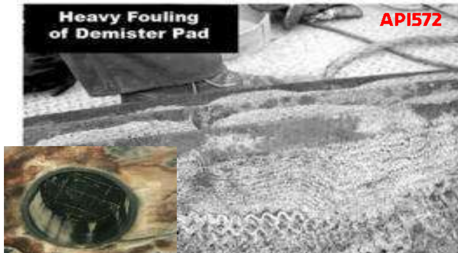
Figure B.39—Fouled Demister Pads
