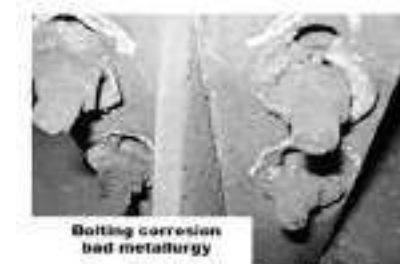
Figure B.48—Hardware Corrosion
